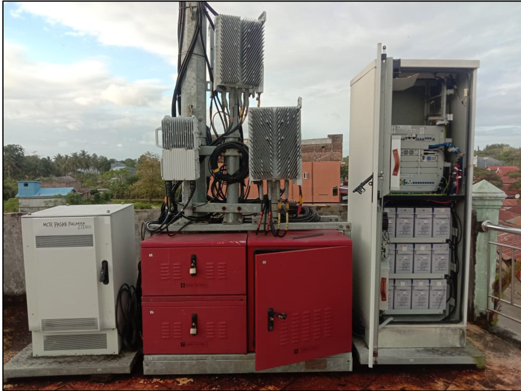
Gambar 4.2 Tower BTS rooftop Pasar Palakka Kab. Bone
