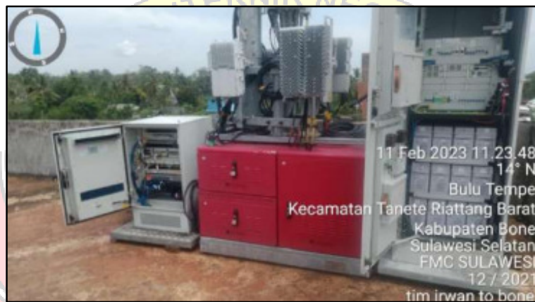
Gambar 2.16 Komponen Telekomunikasi Tower BTS Rooftop Palakka
