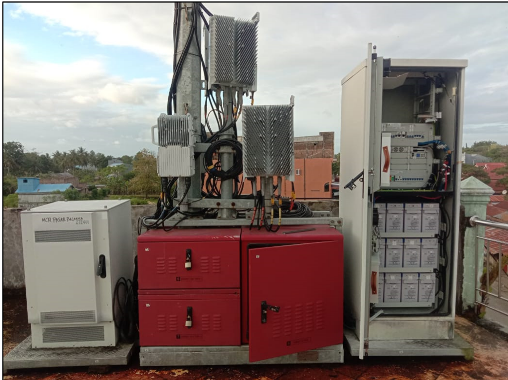
Gambar 2.2 Tower BTS rooftop Pasar Palakka Kab. Bone
