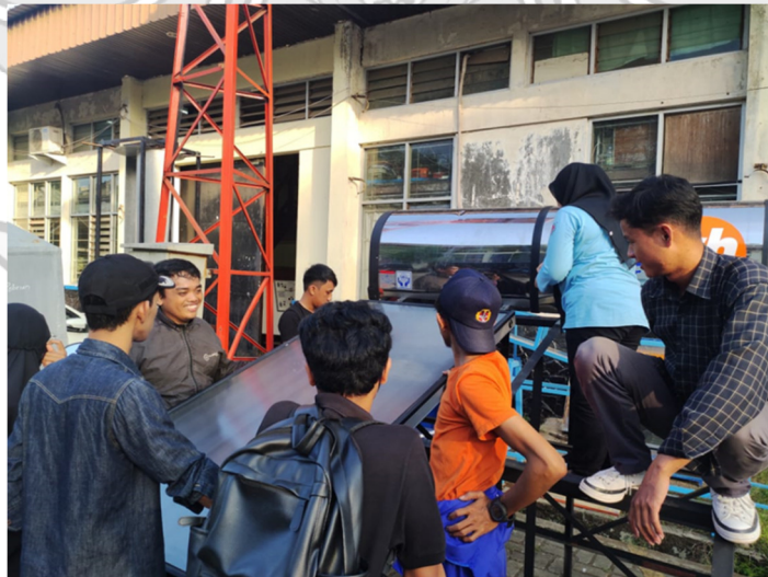
Lampiran 7 Pemasangan Solar Water Heater
