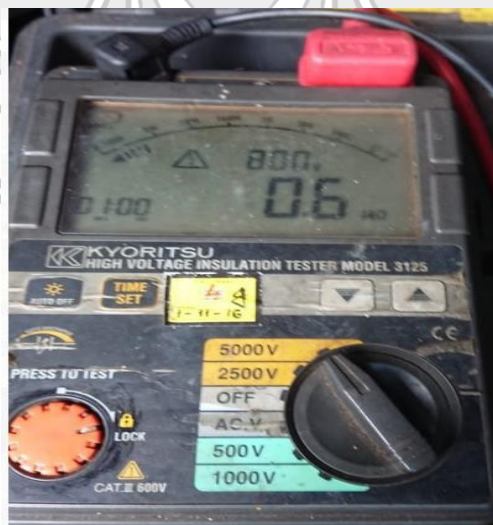
Gambar 4.14 pengukuran phase T 11,5 kV (Sumber: General Electric #1 ULPLTG Tello)
