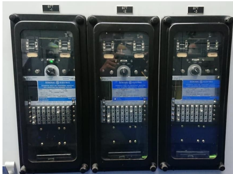
Gambar 4.9 Rele 87T (1), 87T (2), 87T (3) (Sumber: Local Control General Electric #1 ULPLTG Tello)
