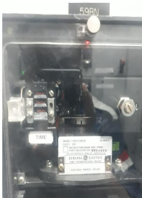
Gambar 4.10 Kondisi fisik Rele Ground Fault ULPTG Tello (Sumber: Local Control General Electric #1 ULPLTG Tello)
