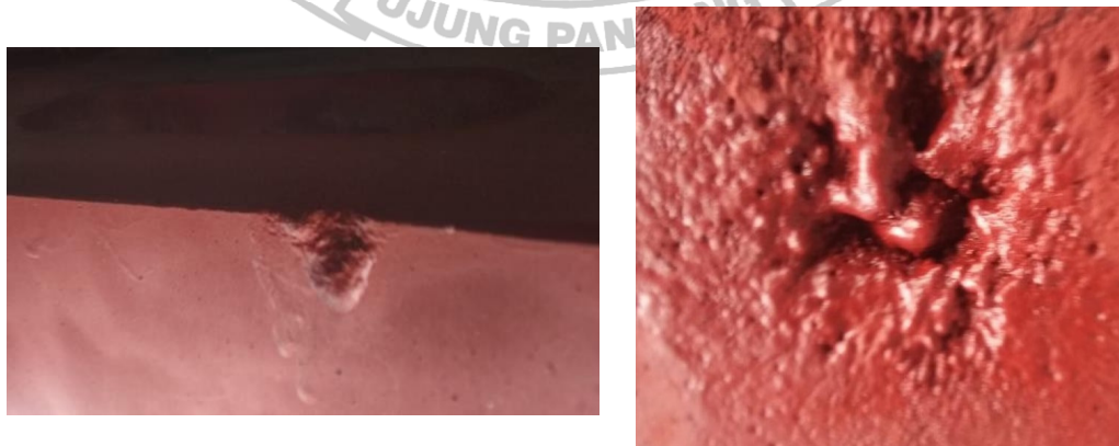
Gambar 4.15 Kebocoran Isolasi Busbar 11,5 (Sumber: General Electric #1 ULPLTG Tello)
