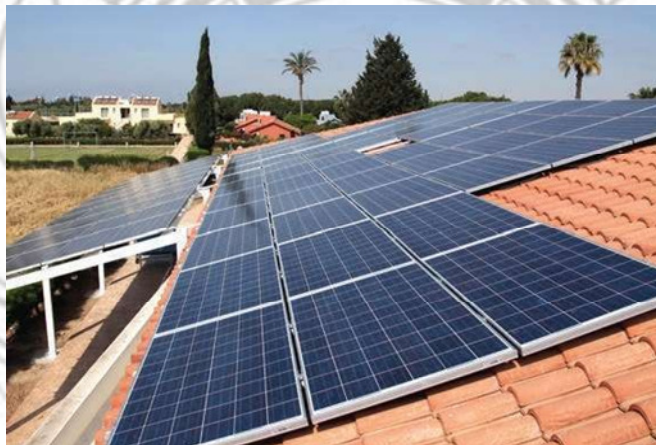
Gambar 2.5 Panel Surya (Sumber: Sanspower, 2020)
