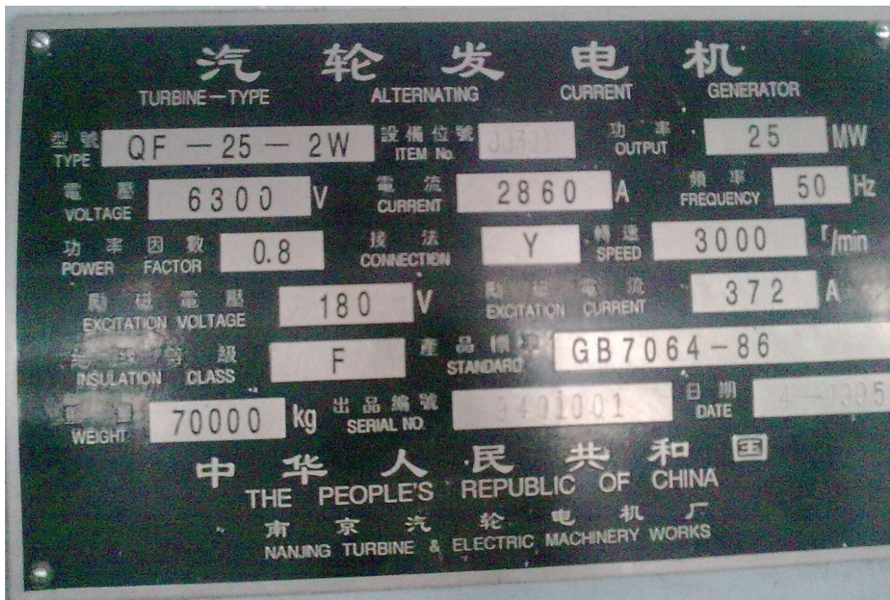
Name plate Generator PLTU BTG PT Semen Tonasa
