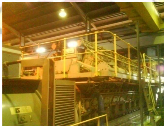
Gambar 2.7 Mirrless Blackstone Diesel Generator (MBDG)
