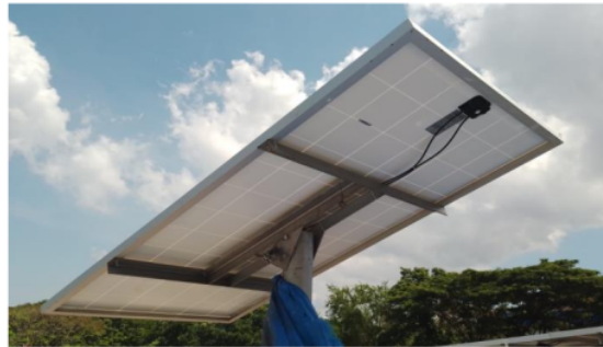
Figure 4. 375 Wp Solar Panel
