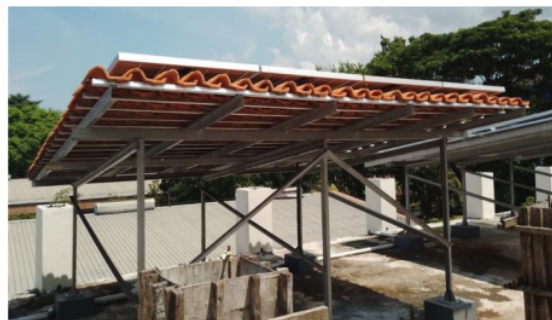
Figure 7. 3 kWp Solar Panel-3
