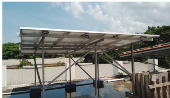
Figure 5. 3 kWp Solar Panel-1
