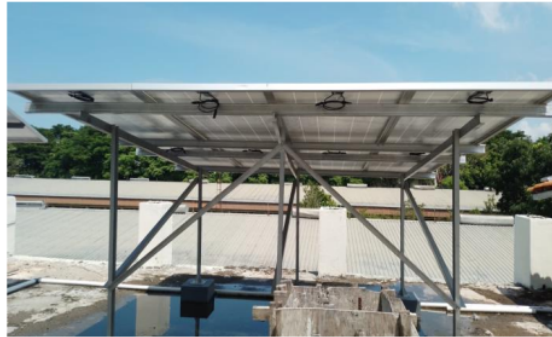
Figure 6. 3 kWp Solar Panel-2
