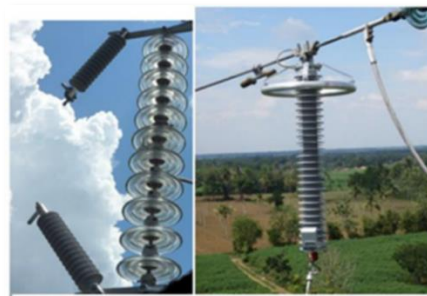
Gambar 3 Transmission Line Arrester (TLA) [6]
