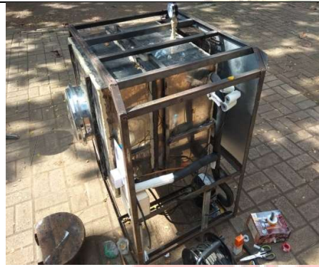
Rangkaian pipa-pipa refrigerasi
