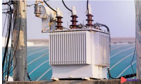
Gambar 2.2. Transformator Step Down
