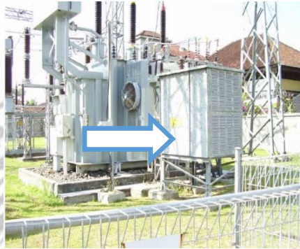
Gambar 14 Netral Ground Resistant (NGR)
