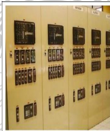
Gambar 10 Panel Kontrol Rele
