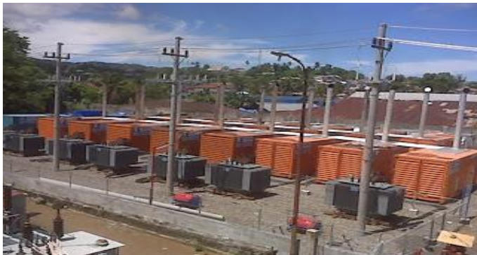
Image: Diesel-fired power plants in Bitung, North Sulawesi, Indonesia . Photo courtesy of putramjl.blogspot.co.id.
