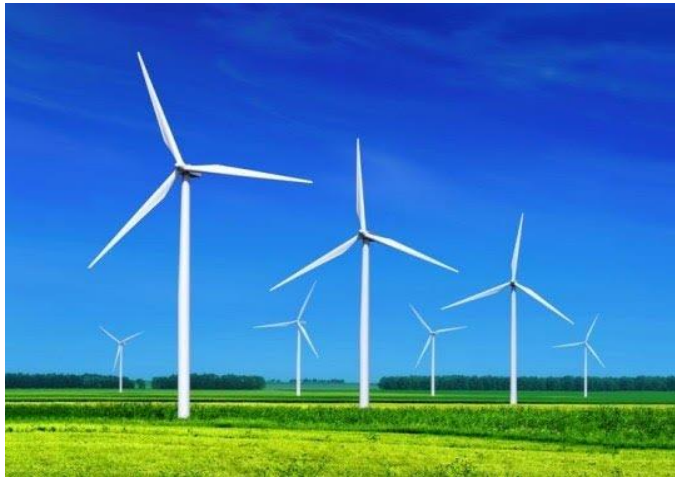
Image: Wind power plant in United Kingdom, Photo: courtesy of tileenergy.uk.
