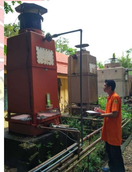
(b) Area Cooling Tower
