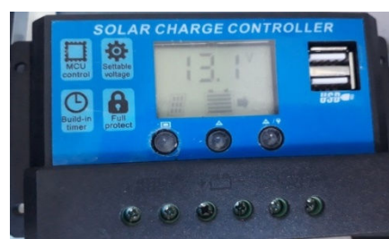
Gambar 7. Baterai Charge Regulator (Controller)
