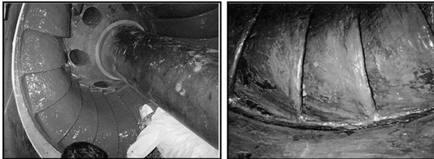
Gambar 2. 12 Contoh Kerusakan Material Runner Akibat Kavitasi (Sumber : https://repository.its.ac.id/ )
