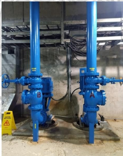
Gambar 2. 2 Drainage Pump (Sumber : PLTA Bakaru)
