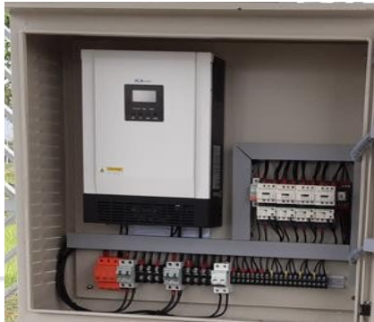
Gambar 4. 13 Electrical Panel Box MOV
