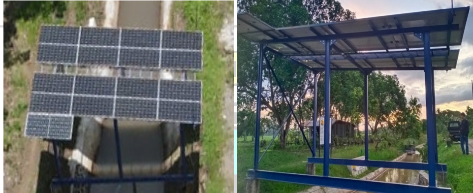
Gambar 4. 22 Mounting System PV Array PLTS Off Grid Pamukkulu'
