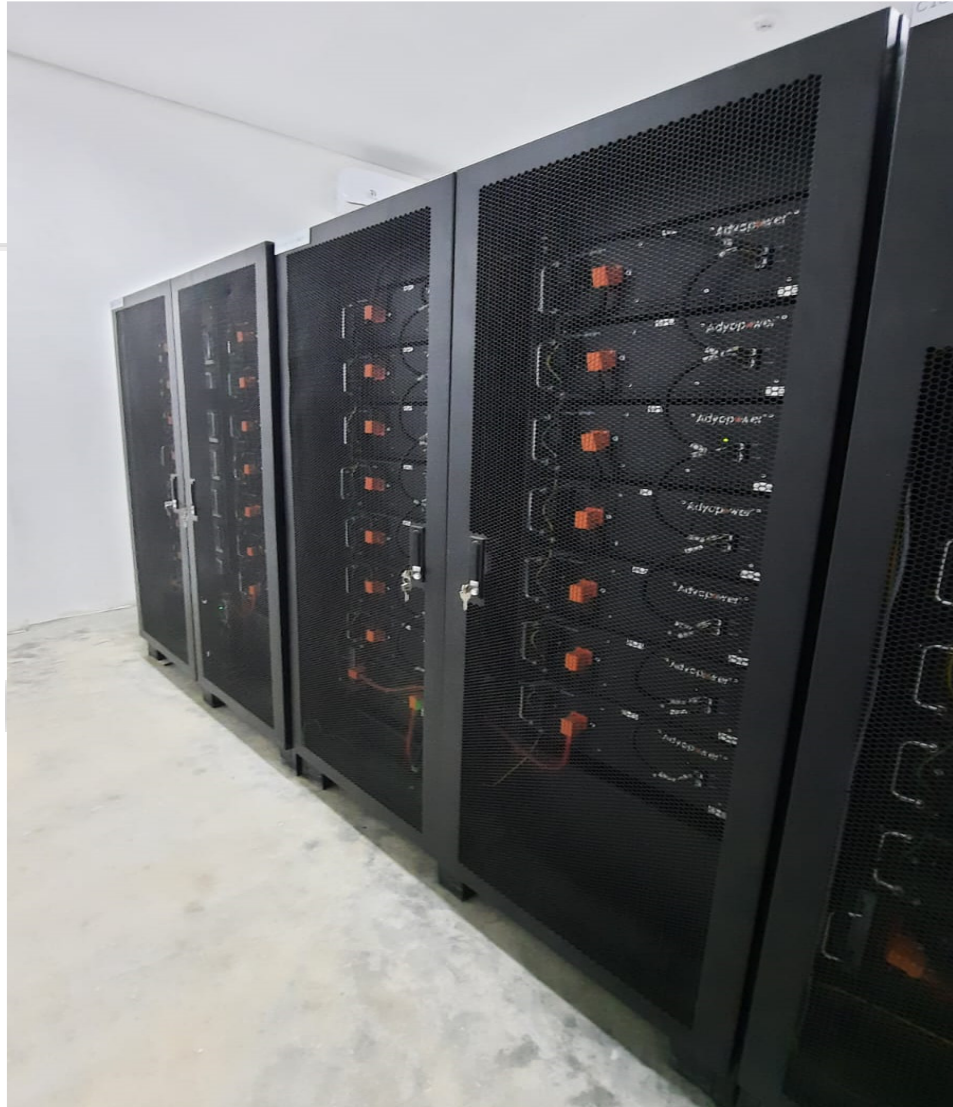
Gambar 2.4 Baterai Lithium Iron Phosphate ( \text{LiFePO}_4 ) PLTS Hybrid Selayar 1300 kWp
