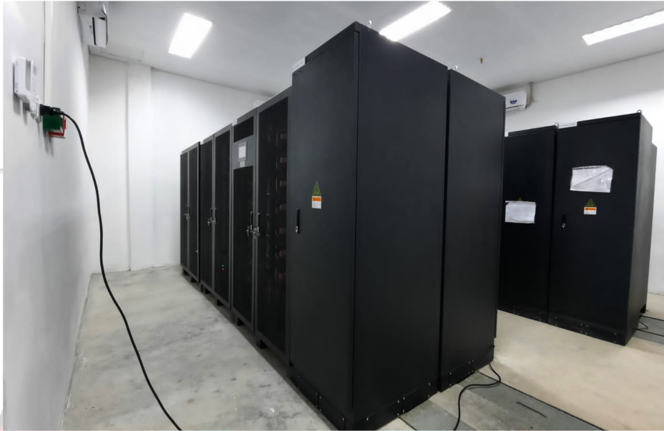
Gambar 3.1 Baterai PLTS Hybrid Selayar 1300 kWp
