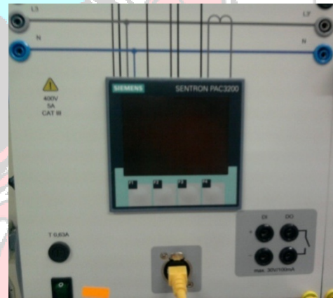
Three Phase Meter
