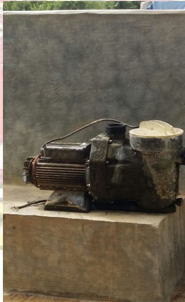
Gambar 28. Pompa Cooling Pad
