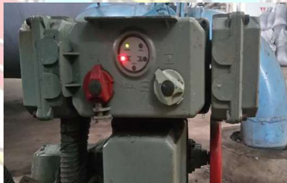
Gambar 2.17 Motor Operated Valve sealing Sumber : PLTU Barru.
