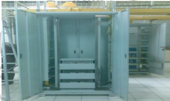
Gambar 2.7 Fiber Termination Management (FTM)
