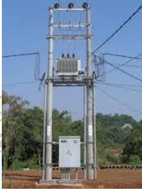
Gambar 1. Gardu transformator Distribusi
