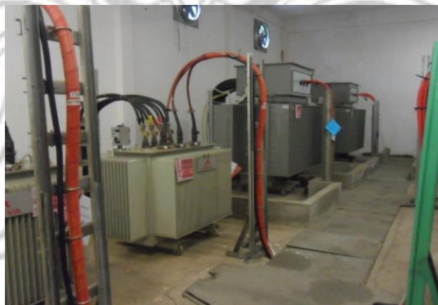
Gambar 6 Transformator TM main power house
