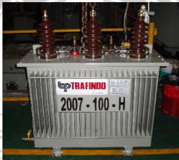
Gambar 8 Trafo Step Down main power house
