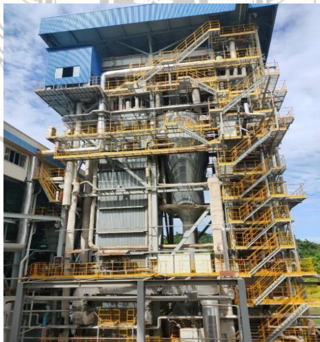
Gambar 2. 6 Boiler CFB (sumber: PLTU Mamuju 2x25 MW)
