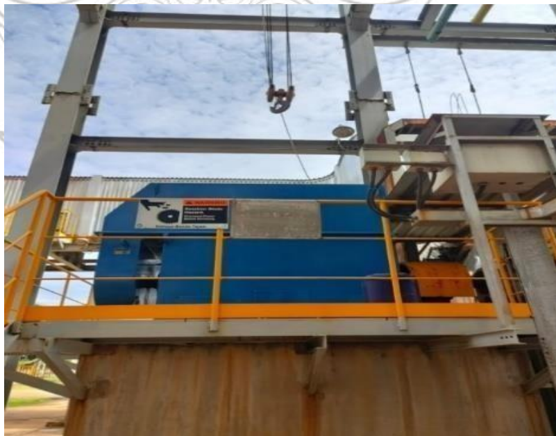
Gambar 2.24 Induced Draft Fan (IDF) (sumber: PLTU Mamuju 2x25 MW)
