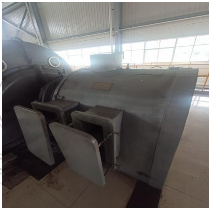
Gambar 2. 23 Main Exciter Generator PLTU Mamuju 2x25 MW
