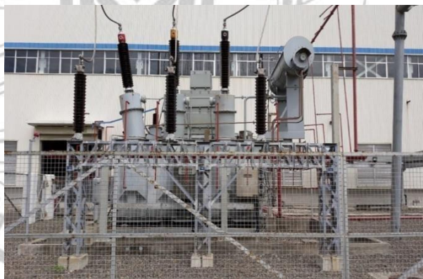
Gambar 2. 24 Main transformator PLTU Mamuju 2x25 MW
