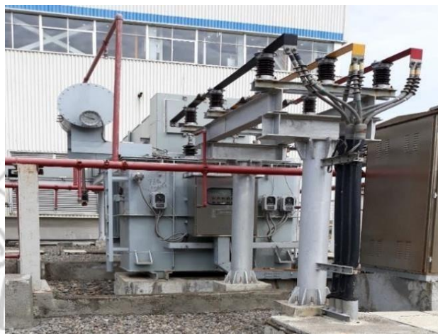
Gambar 2. 25 Auxylary Transformator PLTU Mamuju 2x25 MW
