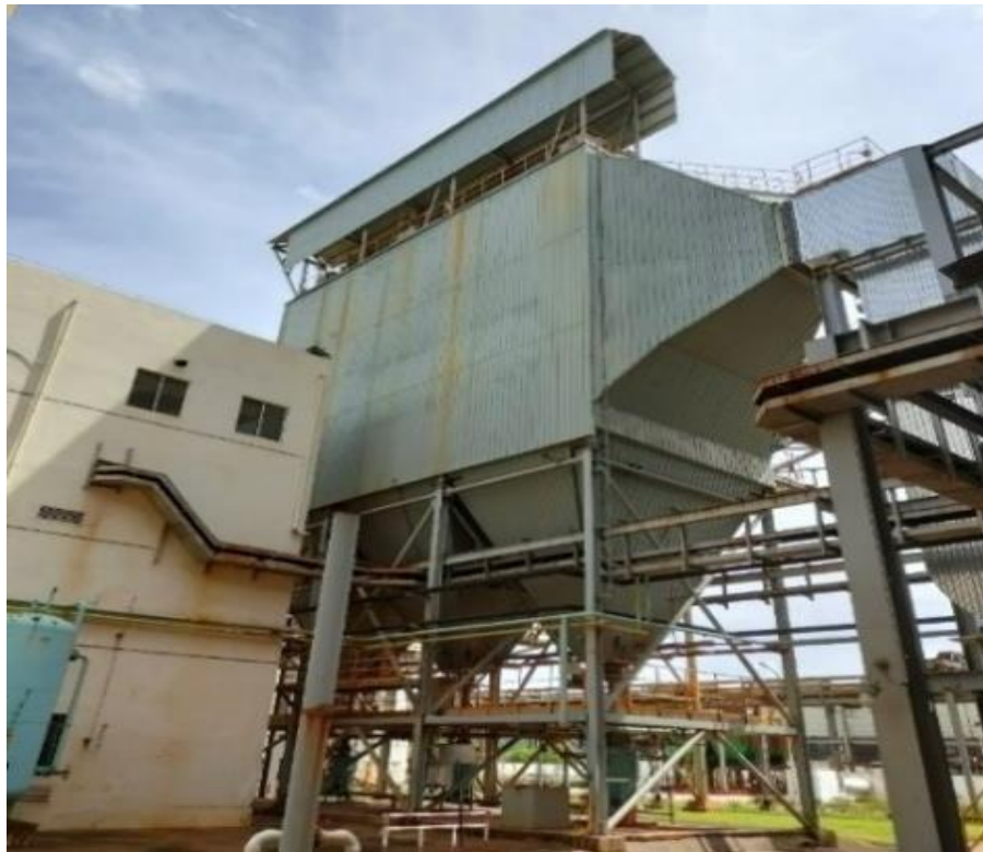
Gambar 2. 19 Electro Static Precipitator (ESP) (sumber: PLTU Mamuju 2x25 MW)
